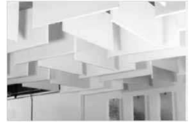
Example of baffles in the ceiling of a machine shop.
